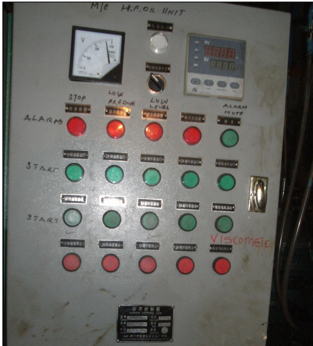
Figure 6: Fuel unit control panel
