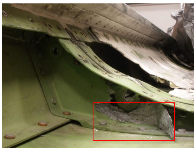
Figure 5: Outboard auxiliary track attachment corrosion
