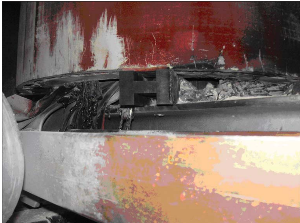
Figure 16: Localised fire damage on number four transformer centre coil
