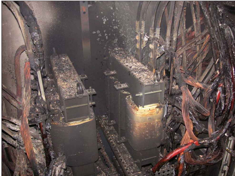
Figure 17: Burnt out upper section of the choke cabinet showing extra cables
