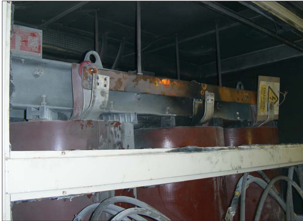
Figure 7: Inside number four transformer cabinet
