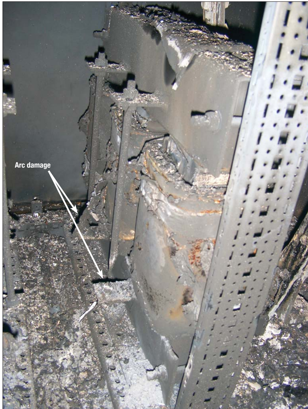
Figure 18: Burnt out lower section of the choke cabinet showing arc damage
