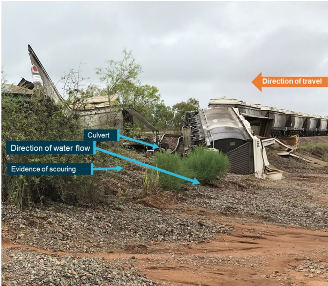
Figure 11: Evidence of scouring on the downstream (outlet) side
