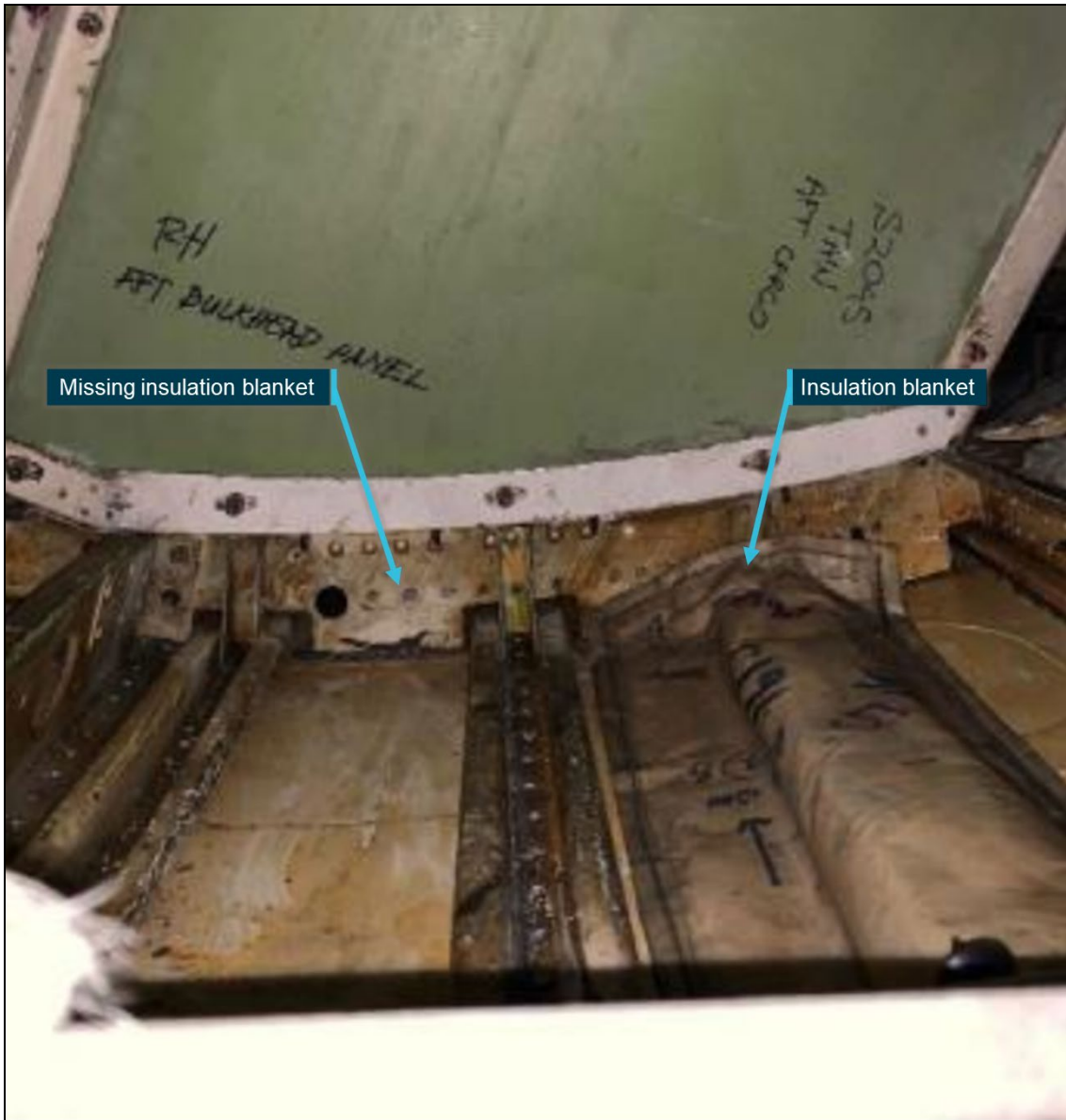
Figure 2: Missing insulation blanket aft cargo bay
