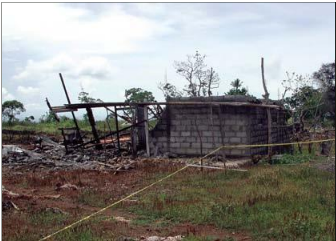
FIGURE 6: Partially constructed house struck by the aircraft during the impact sequence
