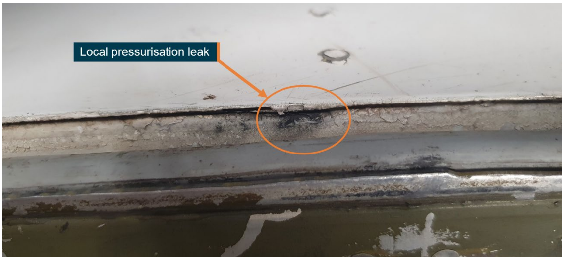
Figure 6: Indication of a local pressurisation leak
