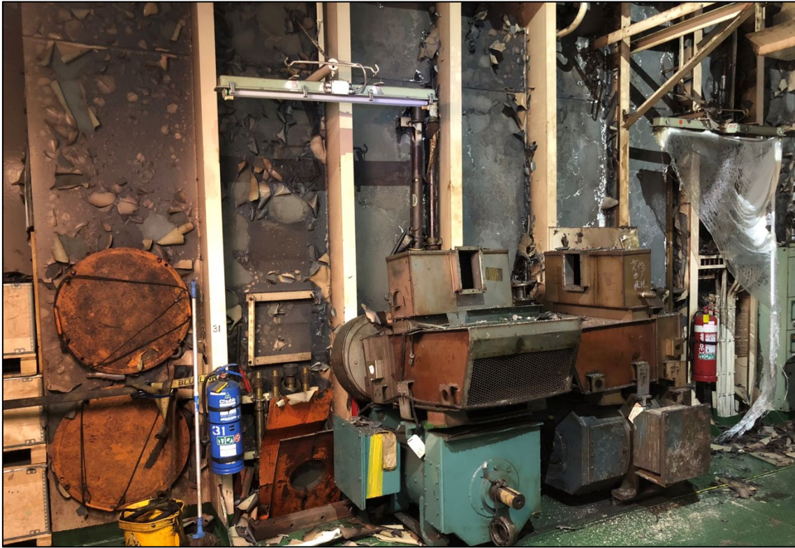
Figure 17: Heat damage to engine room forward bulkhead
