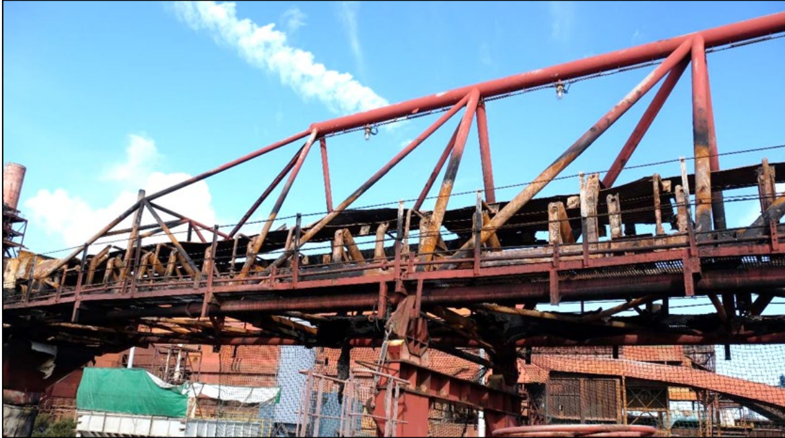
Figure 16: Fire damage to the SUL system boom
