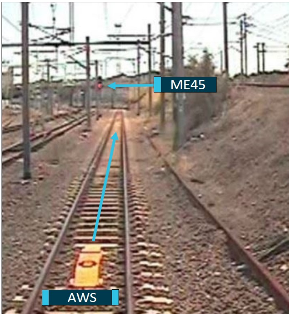
Figure 3: AWS magnet and signal ME45 displaying a red (stop) aspect
