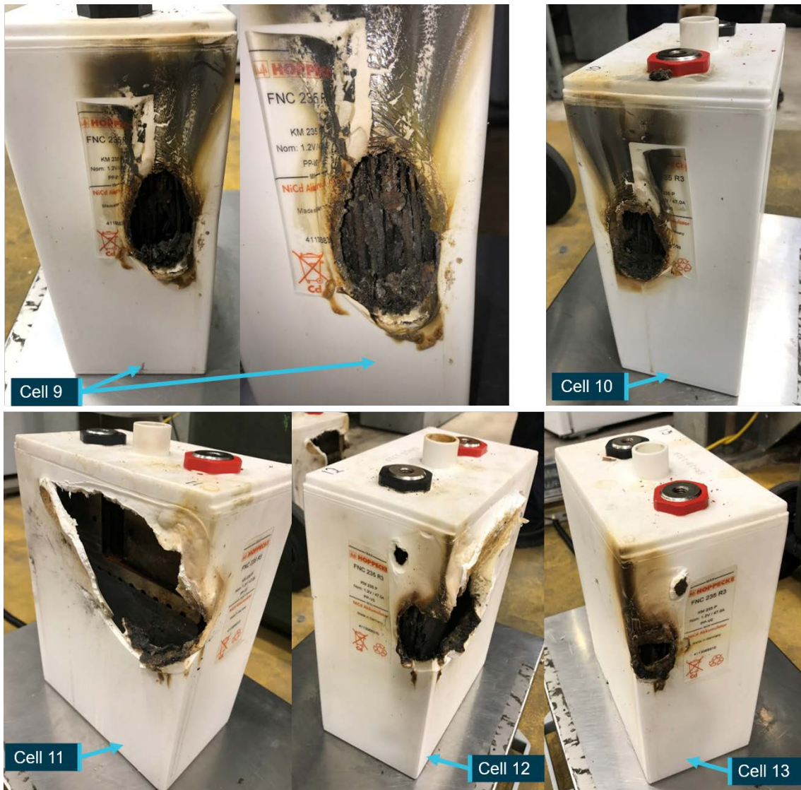
The image shows the damage to the cell casings for batteries 9 to 13. Cell casings for batteries 11 and 12 were fused and required mechanical separation to remove from the battery compartment. Source: OTSI
