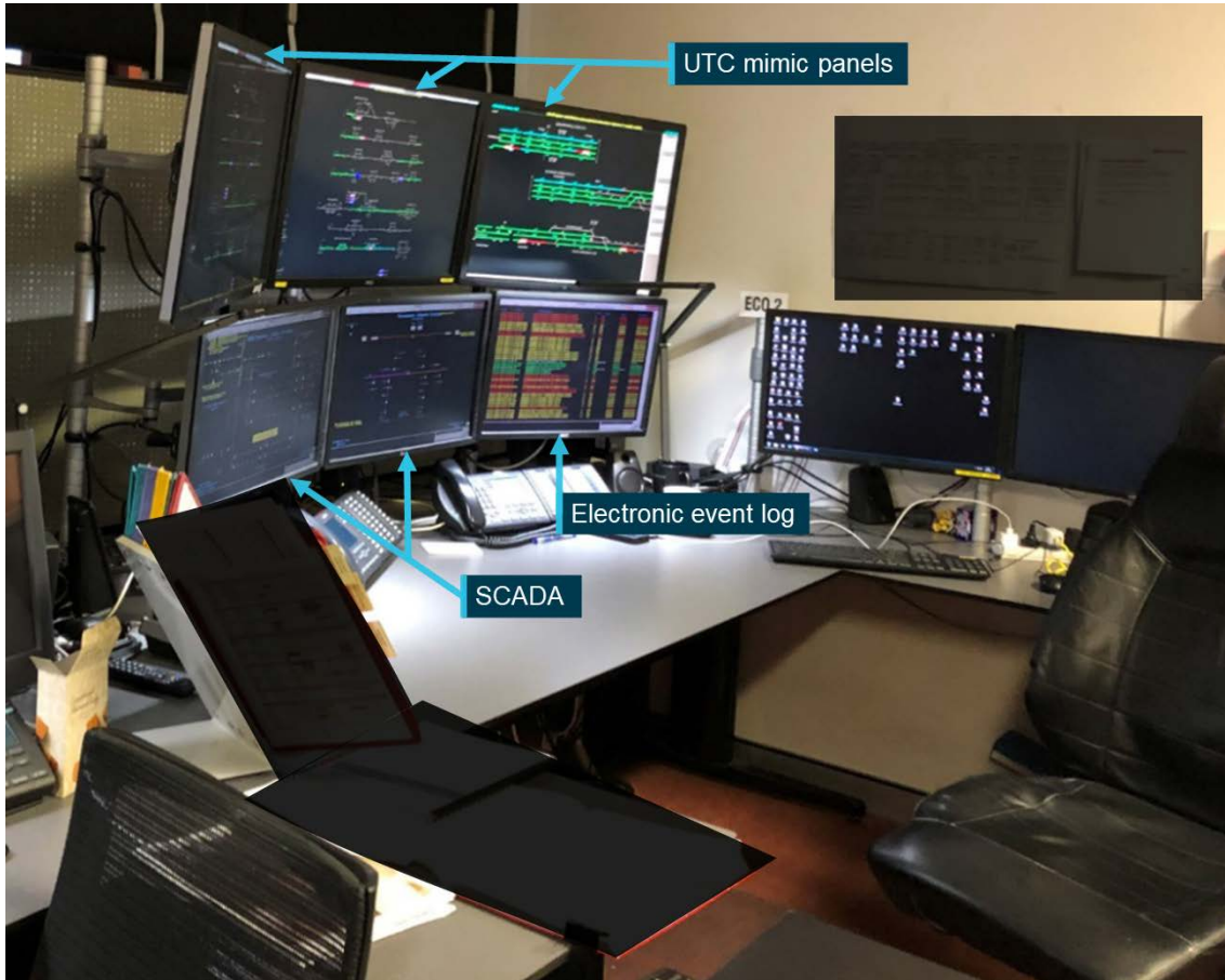
Figure 14: Electric control operator workstation
