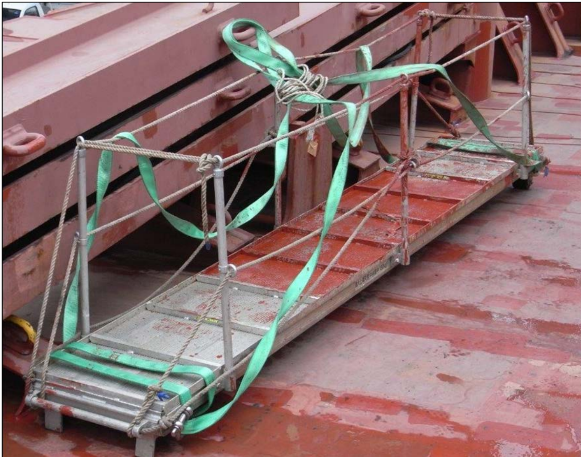
Figure 2: Portable ship’s gangway as rigged for use as the suspended painting platform
