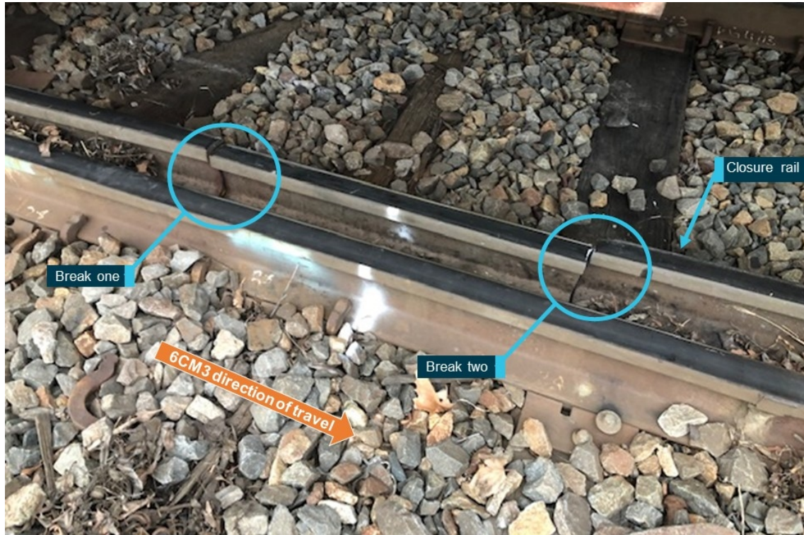
Figure 3: Broken rail segment
