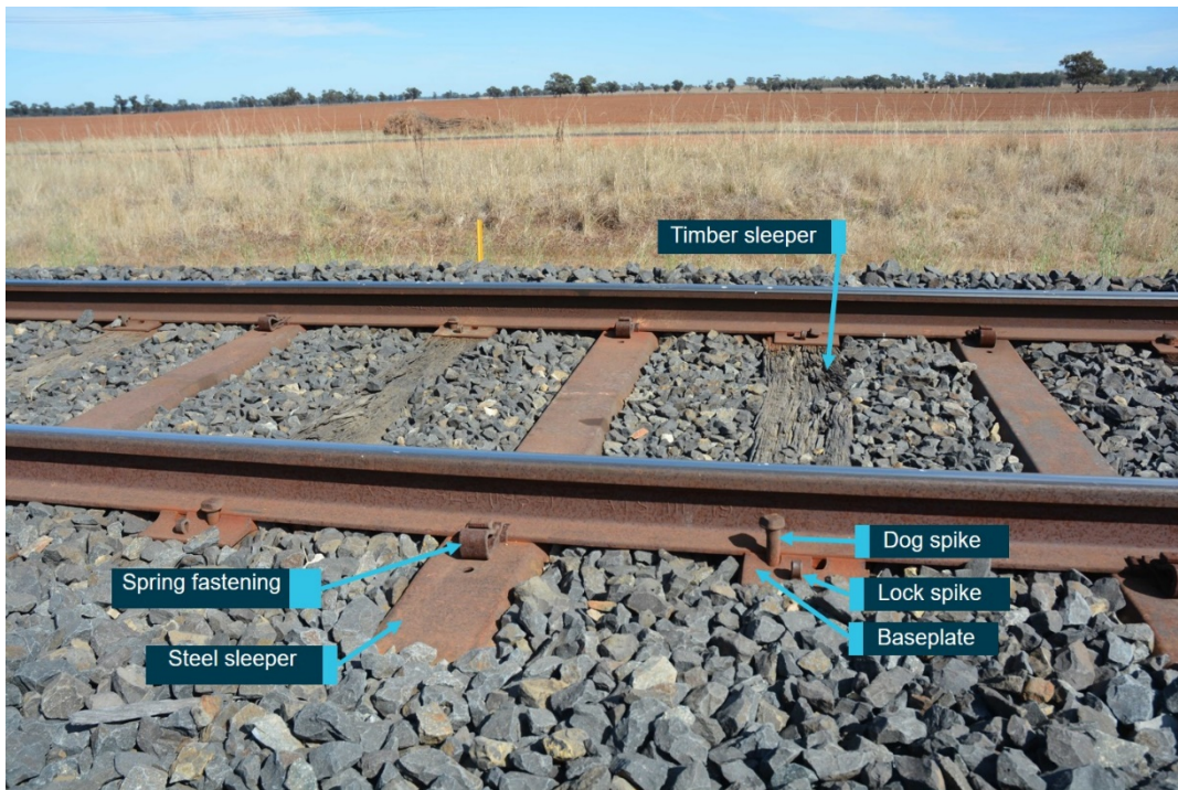
This figure shows the track structure near the derailment at Narwonah. Source: ATSB
