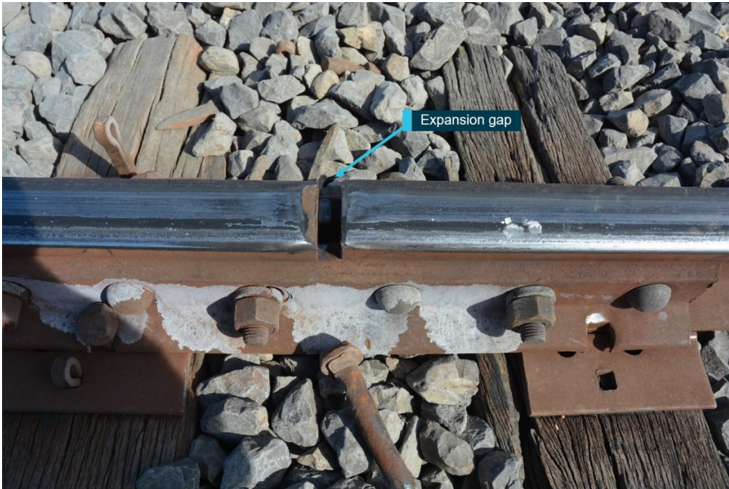
This figure shows the expansion gap at the rail joint on the down rail at 536.989 km. Source: ATSB
