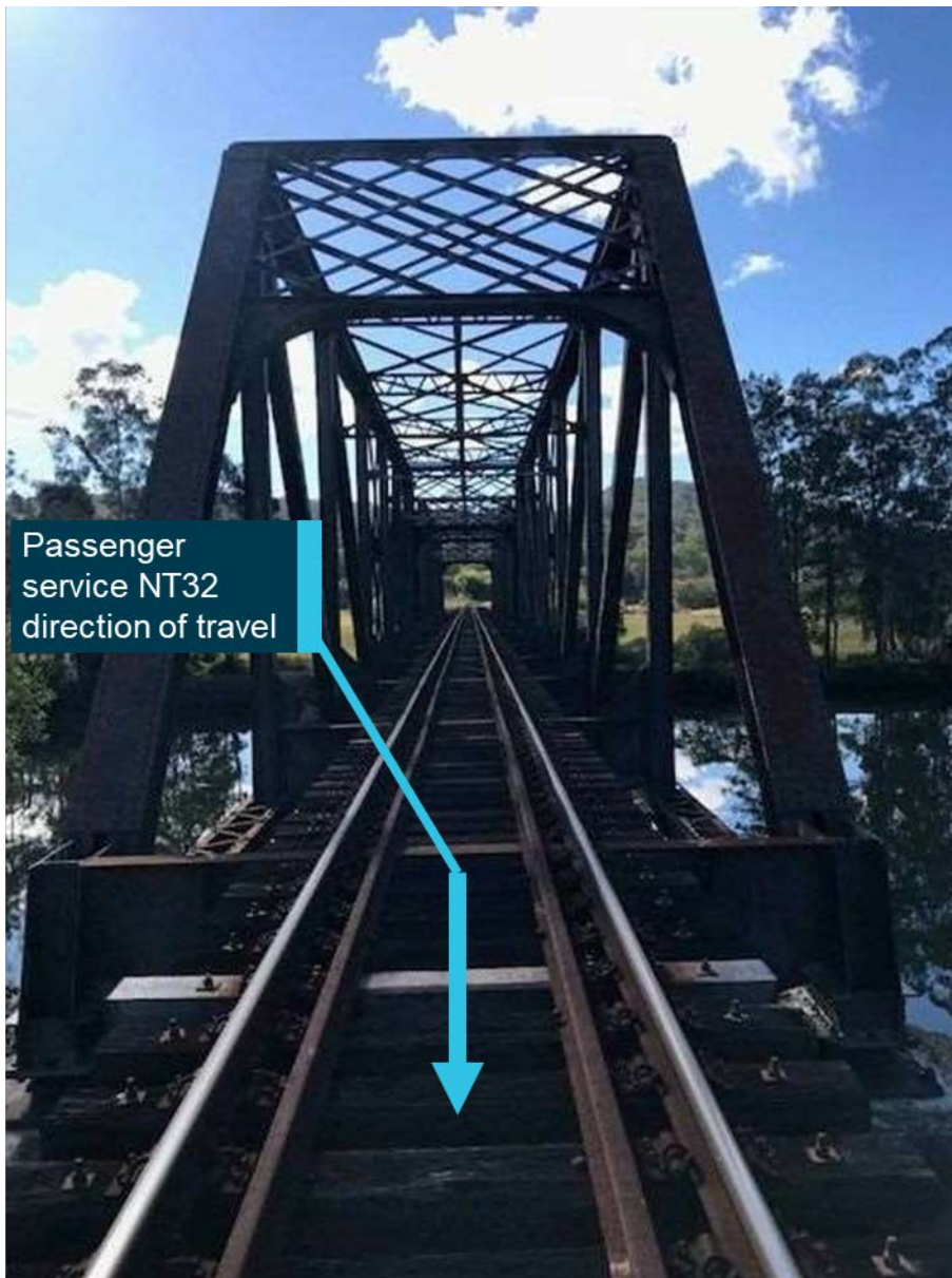
The southern access to the Wilson River Bridge, facing north. This view shows the steel through truss structure that the awning struck. Source: Pacific National
