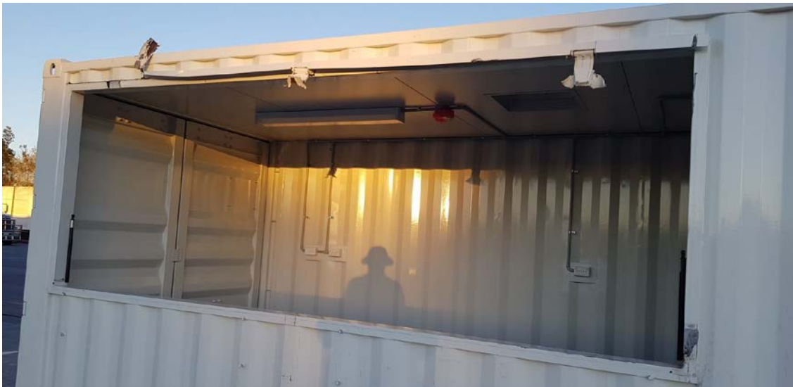
Figure 4: View of the container showing the damage from the missing awning
