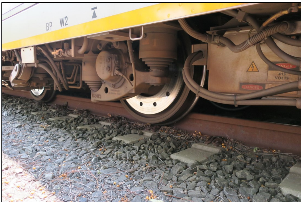
This figure shows the derailed wheels on the bogie on the No.1 end of the fifth car (T6642) (non-platform side).
