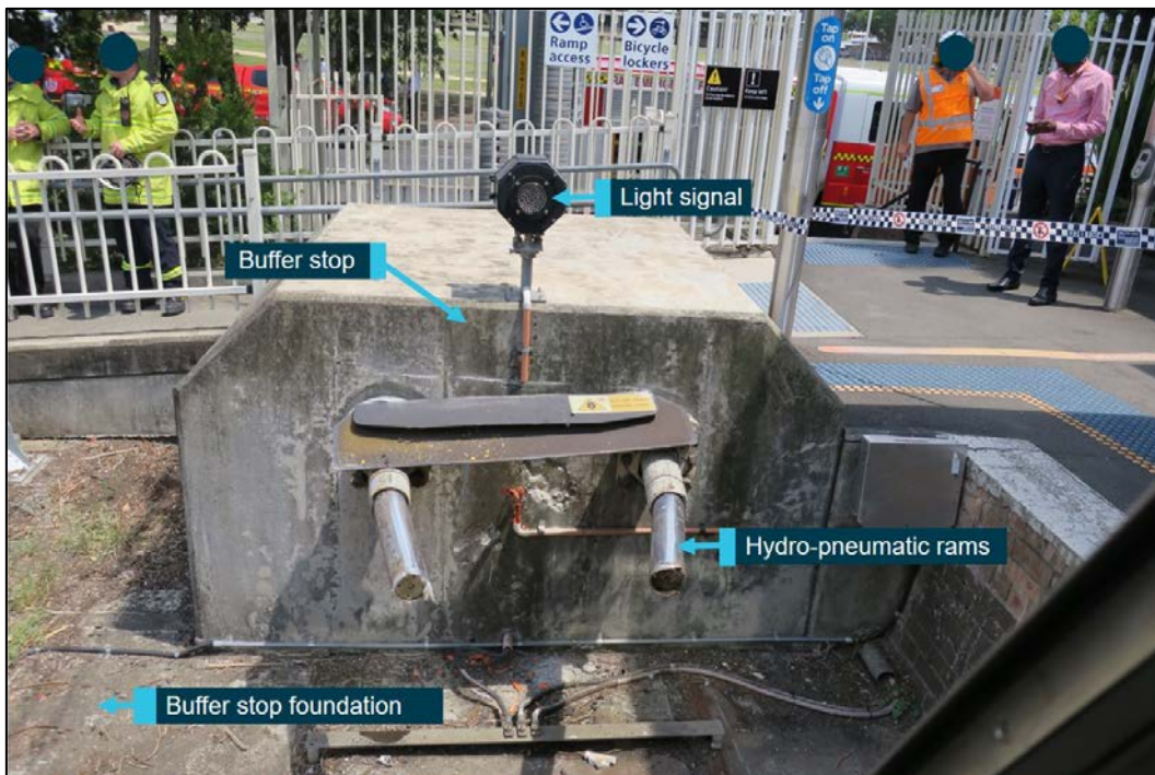
This diagram shows the post-collision damage to the buffer stop on Platform 2, details at Richmond Station, and the light signal attached to the buffer stop. Source: ATSB
