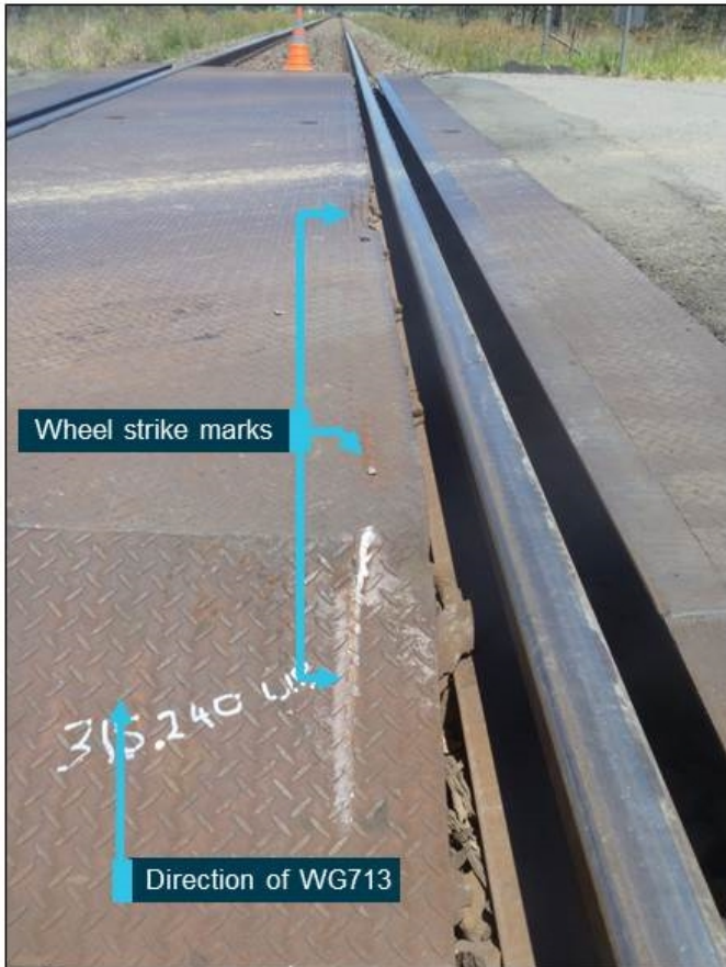
Figure 2: Wheel strike marks on Rosemount Road level crossing road plate
