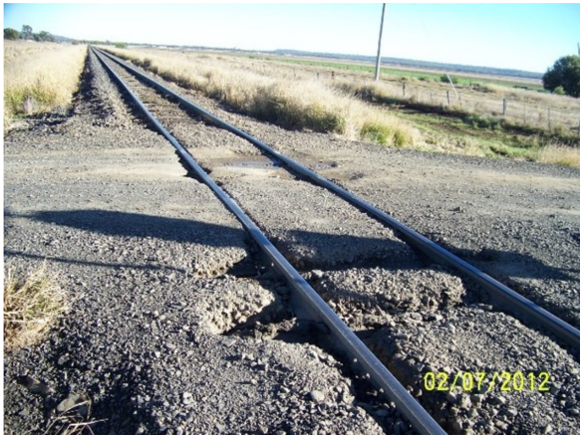
The assessors report recorded that the crossing gravel surface is breaking up and the track is ‘pumping’ and contributing to surface deterioration. Source: QR
