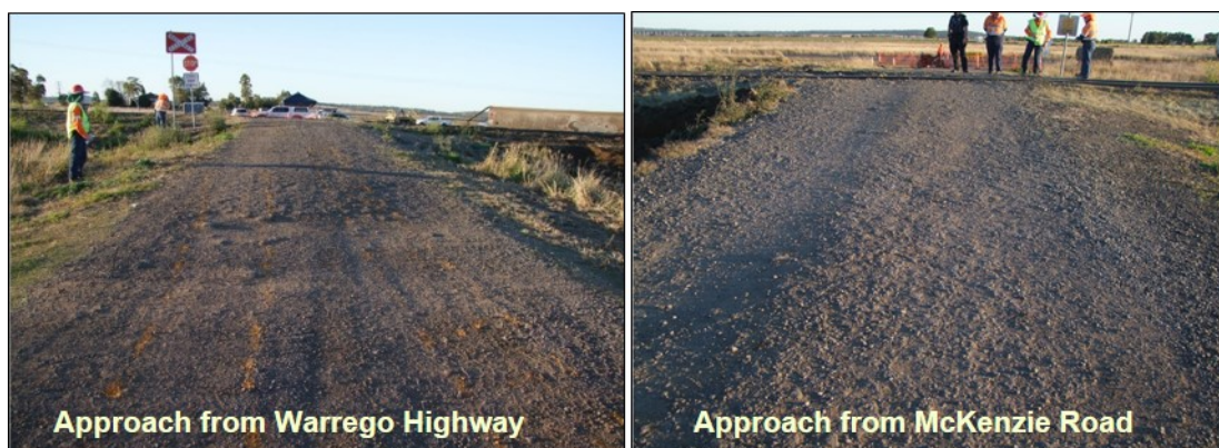
The images show the deteriorated state of the road surface and evidence of wheel furrow marks cut into the road surface. Source ATSB
