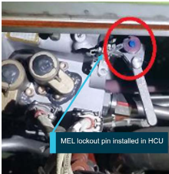
Figure 1: MEL lockout pin installed in thrust reverser hydraulic control unit (HCU)
