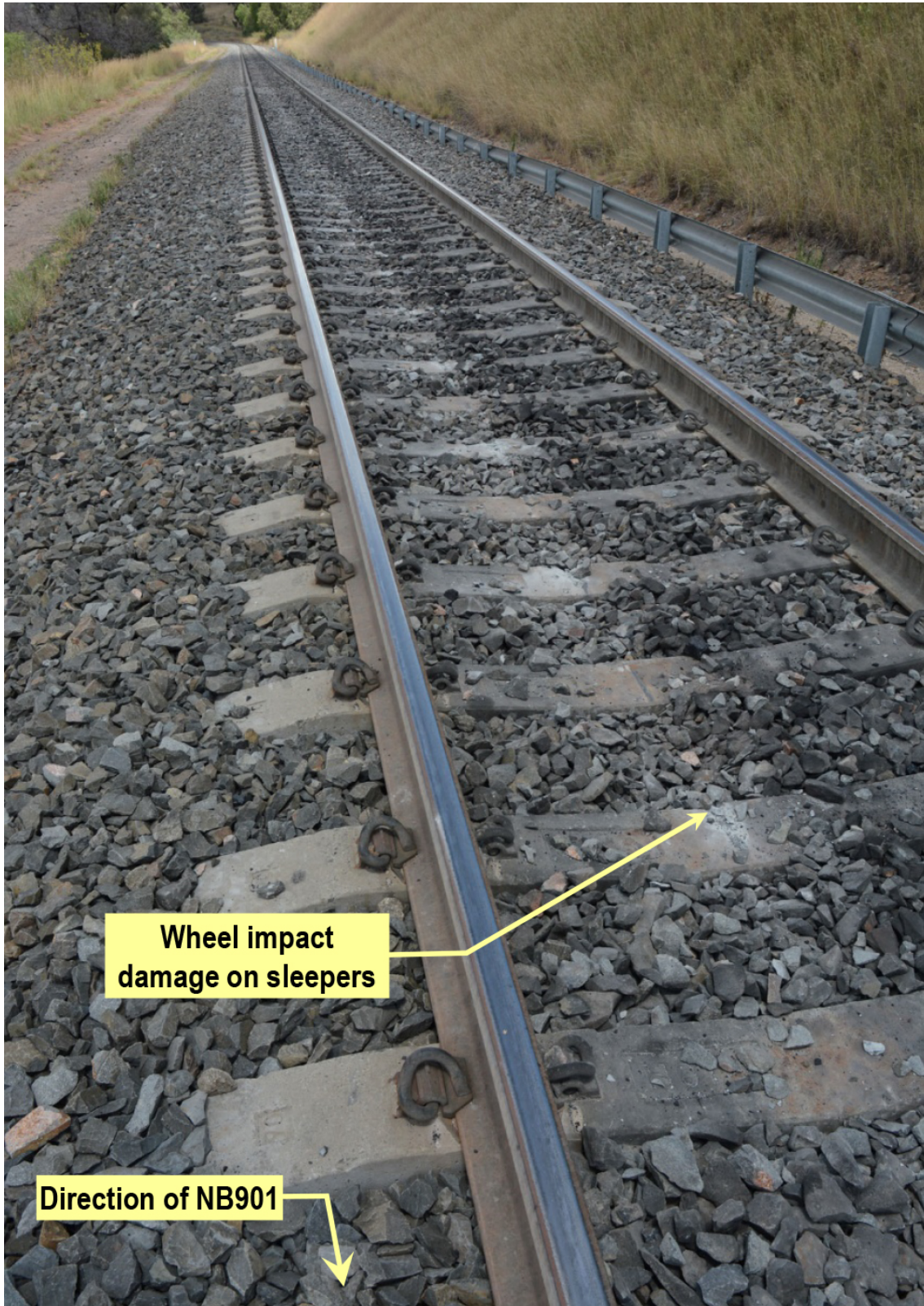
Figure 8: Wheel impact damage on track
