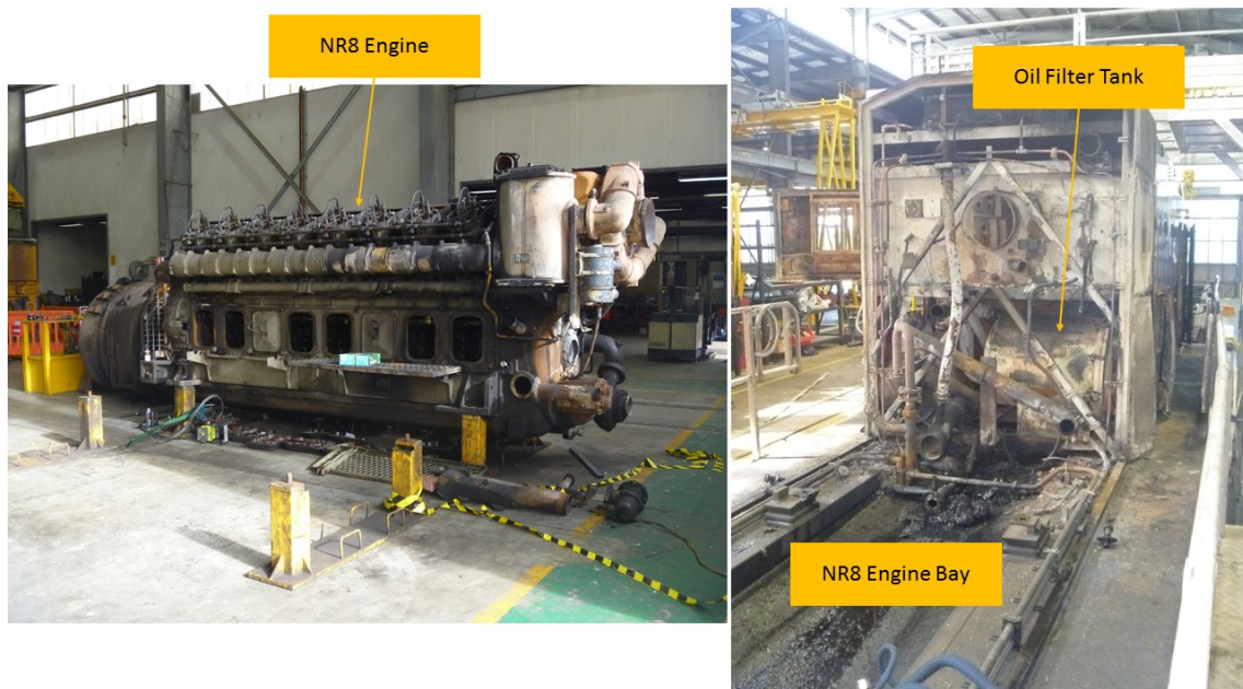
Figure 3: NR8 engine removed from bay (L) and oil filter tank in situ (R)
