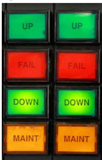
Figure 2: Tower control console hookcable pushbuttons
