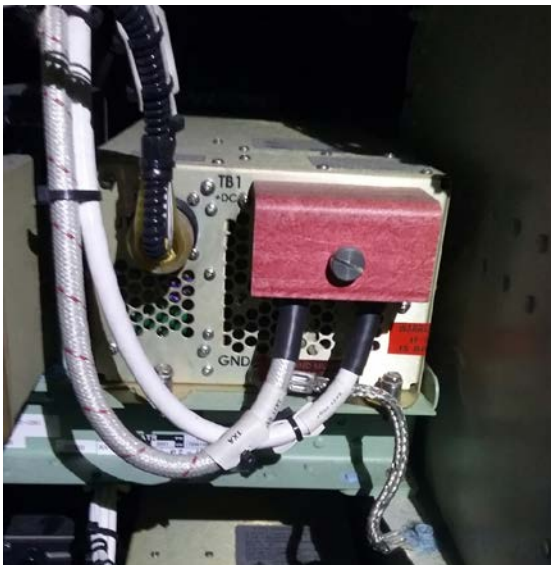
Figure 1: Number one static inverter
