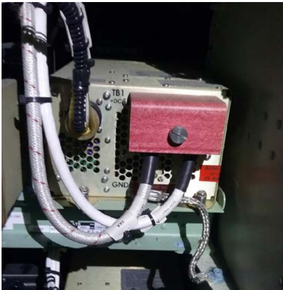
Figure 3: Number one static inverter
