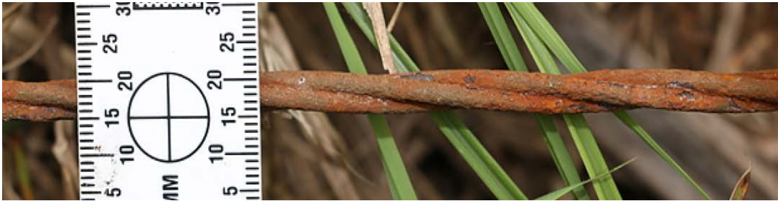
Figure 2: Power cable consisting of three steel wires twisted together (note the rust-like discolouration)
