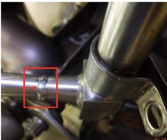
Figure 2: Fractured oil supply line
