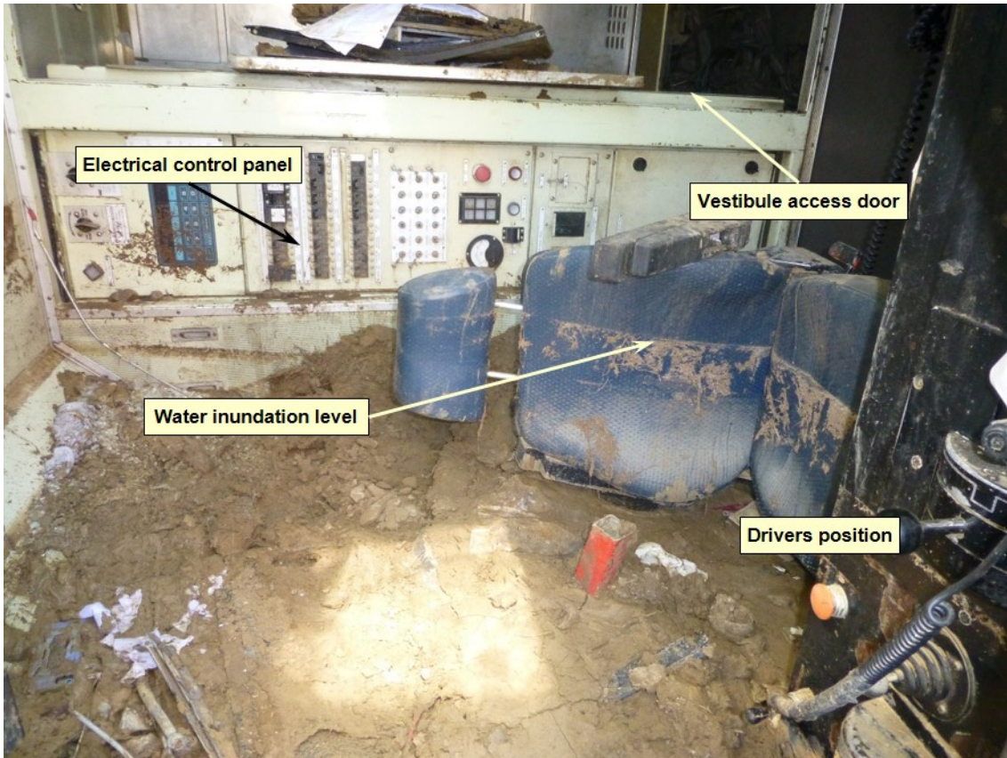
Image showing drivers side seating position and vestibule access door at the rear of the cab post derailment. Floodwaters and sediment entered the locomotive cab to a depth of 600 mm inundating communications and electrical systems. Debris in vestibule door was placed in vestibule during recovery operations. Source: ATSB
