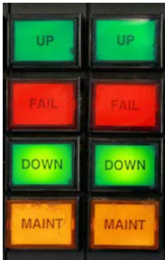
Figure 2: Tower control console cable pushbuttons
