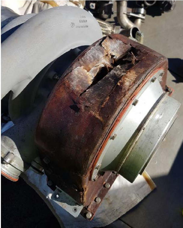
Figure 3: Ruptured plenum duct
