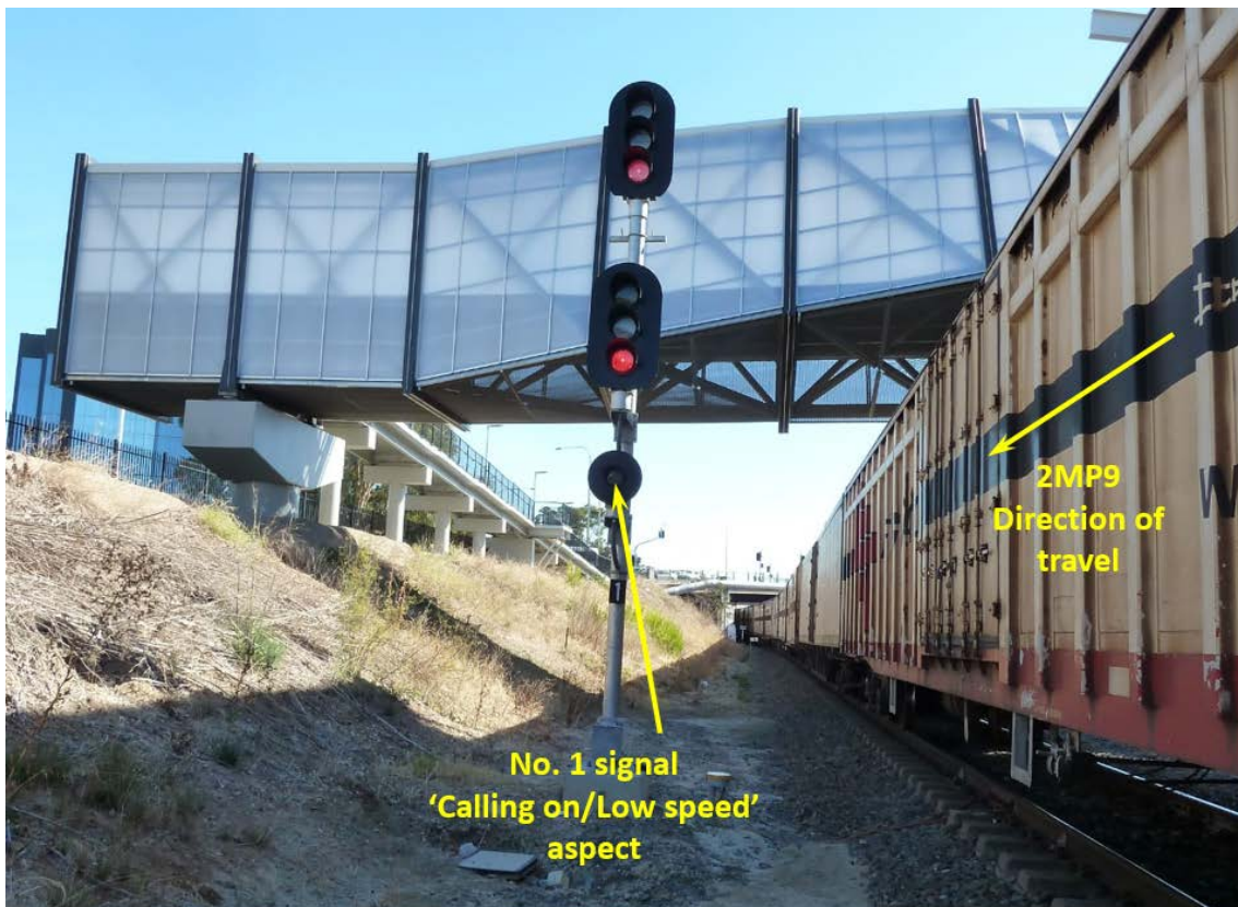
Figure 10: No. 1 signal showing position of Calling on/Low speed aspect
