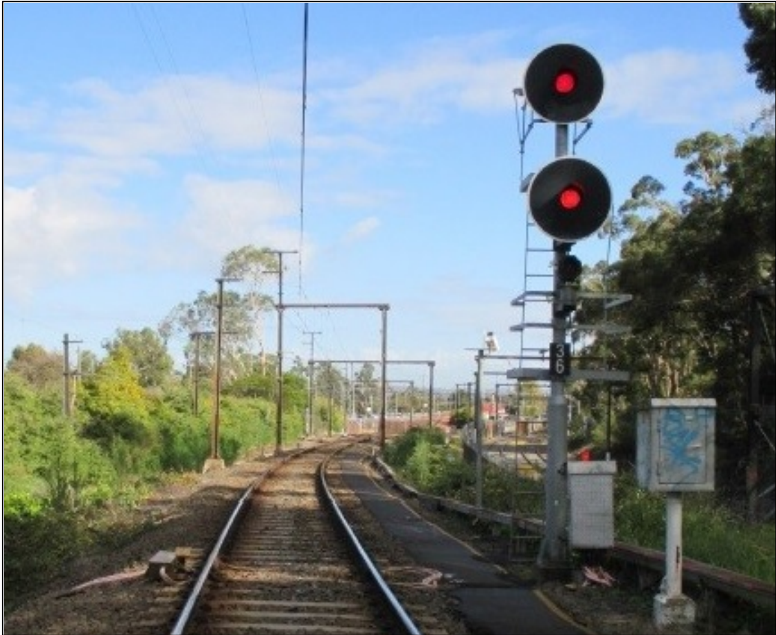
Figure 6: Home arrival signal № 36 at Upper Ferntree Gully
