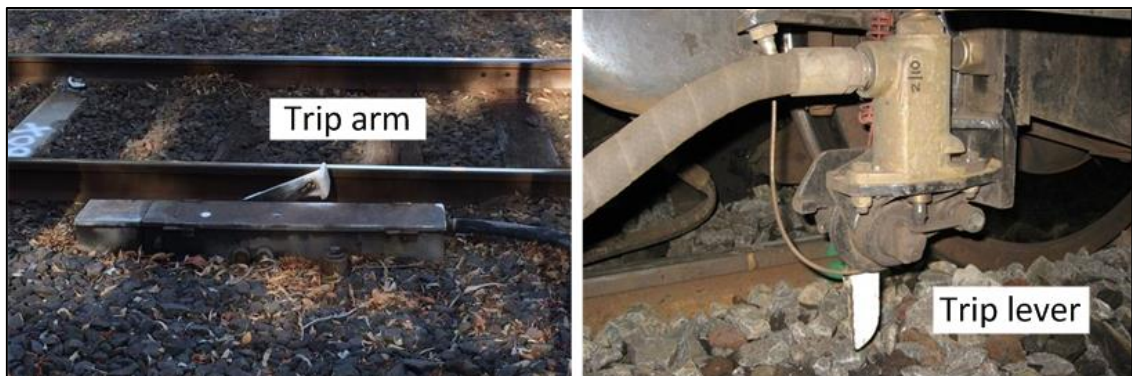
Figure 7: Automatic train stop (left) and trip lever on suburban trains (right)
