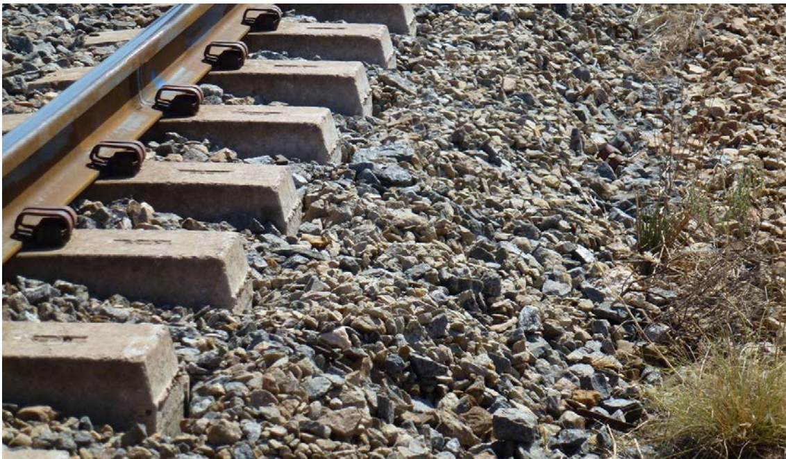
Figure 7: Shoulder ballast and exposed sleeper ends adjacent to the derailment site.
