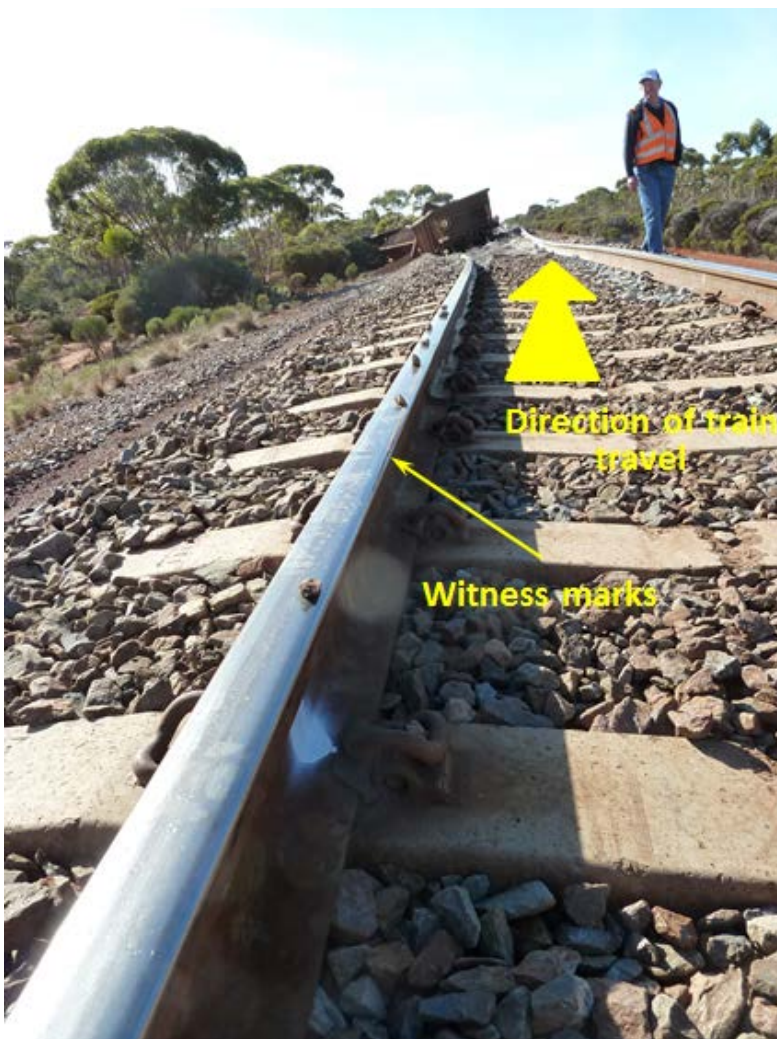
Figure 3: Witness marks caused by a wheel flange at PoD (600.729 km) shown by line of stones on rail head
