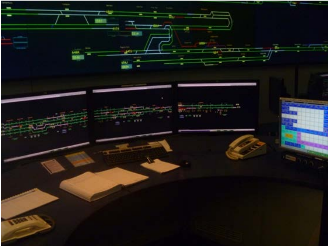
Figure 3: Sydenham signal complex – Revesby control panel
