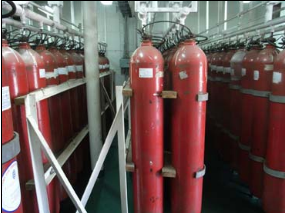
Figure 7: Fixed CO 2 fire extinguishing system
