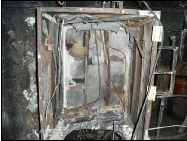
Figure 22: Burnt out telephone booth
