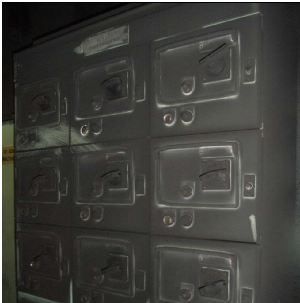
Figure 27: Electrical distribution board with damaged switches directly in line with the hole that had been cut in the deck
