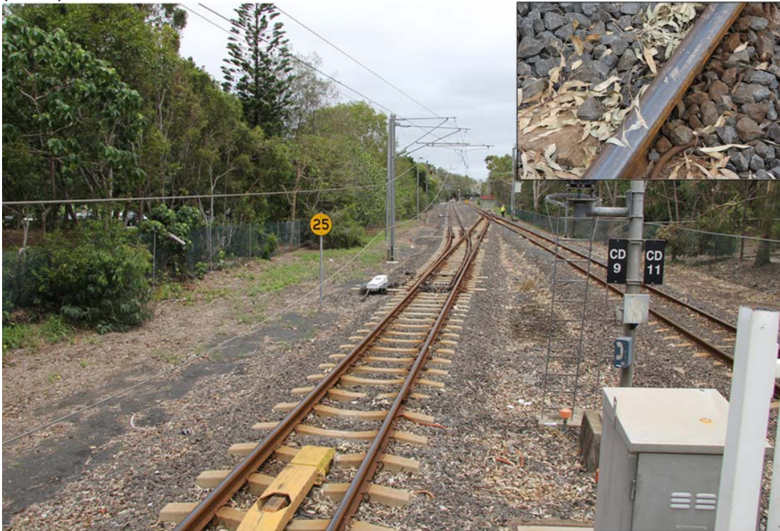
Figure 6: View from Cleveland station platform showing leaf litter about the track and (insert) crushed on the rail head.
