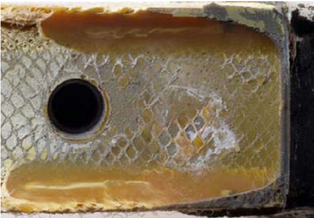
b) Detailed view of the region between the inboard bolthole and spar end
