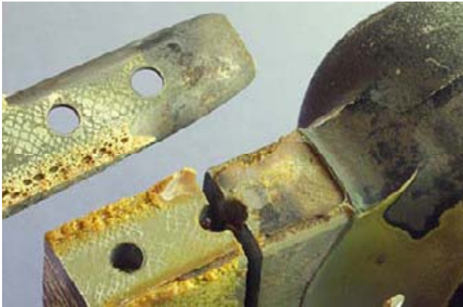
Figure 12: The extent of disbonding between the spar and root fitting, blade s/n 6249A
