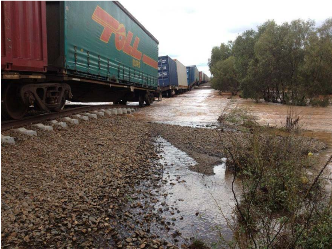
Figure 4: Floodwaters adjacent Roto culvert, viewed in easterly direction toward Roto
