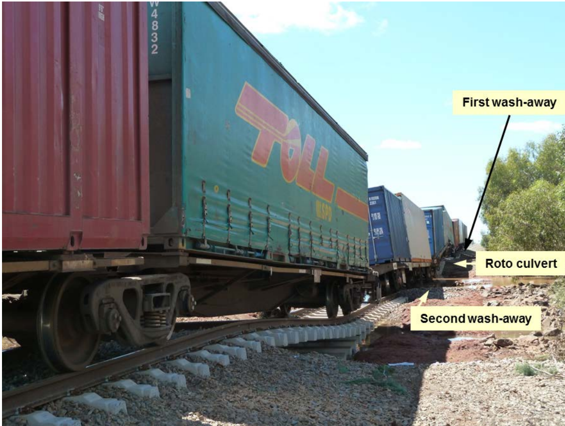
Figure 5: Wash-away damage to track formation adjacent Roto culvert, viewed toward Roto (note the same perspective to Figure 4)
