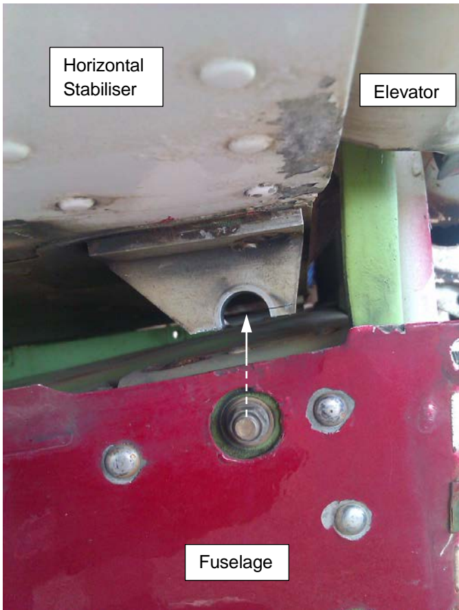
Figure 3: Fractured left bracket, separated from attachment bolt
