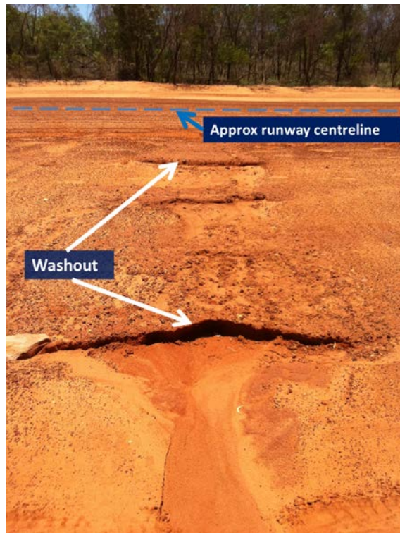
Figure 2: Washout on edge of airstrip
