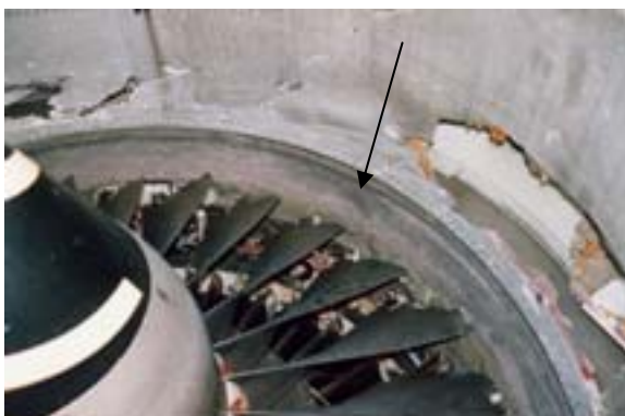
Fig. 5. View of the fan containment shroud showing the released blade impact point.
