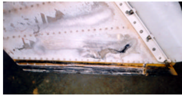
Fig. 20. Area of skin burn-through, with associated thermal damage to the internal honeycomb structure.
