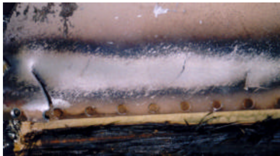
Fig. 19. Closer view of the heated area, showing the development of transverse cracking.
