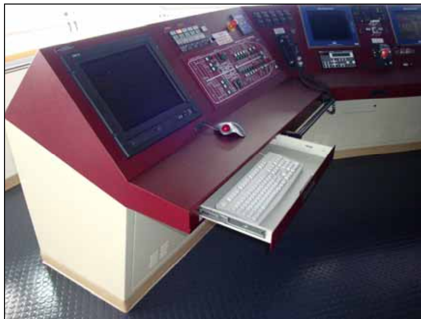
Figure 17: Bridge console inadequately equipped with handrails
