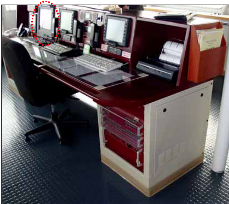
Figure 36: Replay station (integrated in the GMDSS console)
