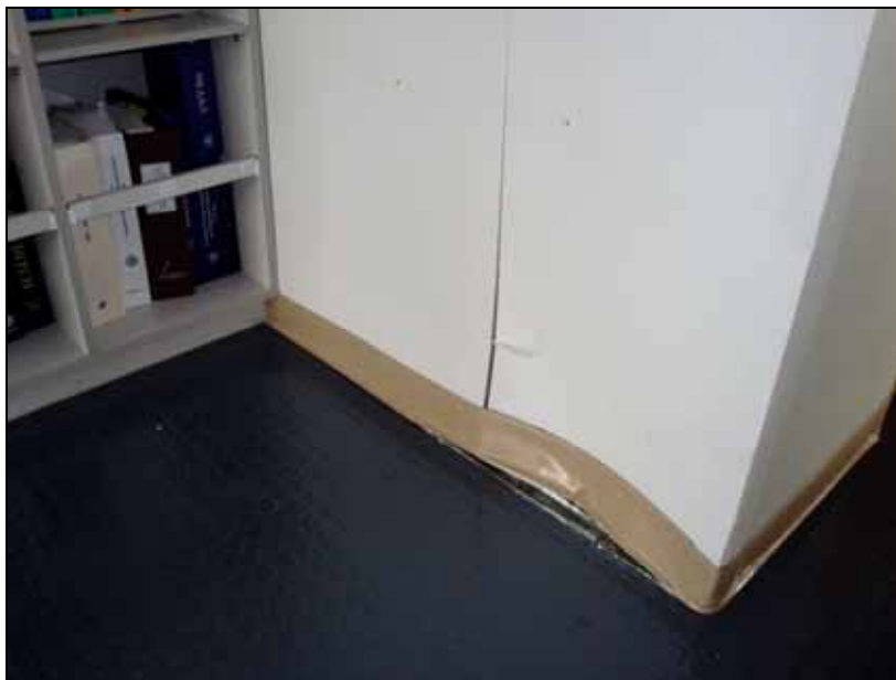
Figure 7: Deformed interior panelling at floor level 17
