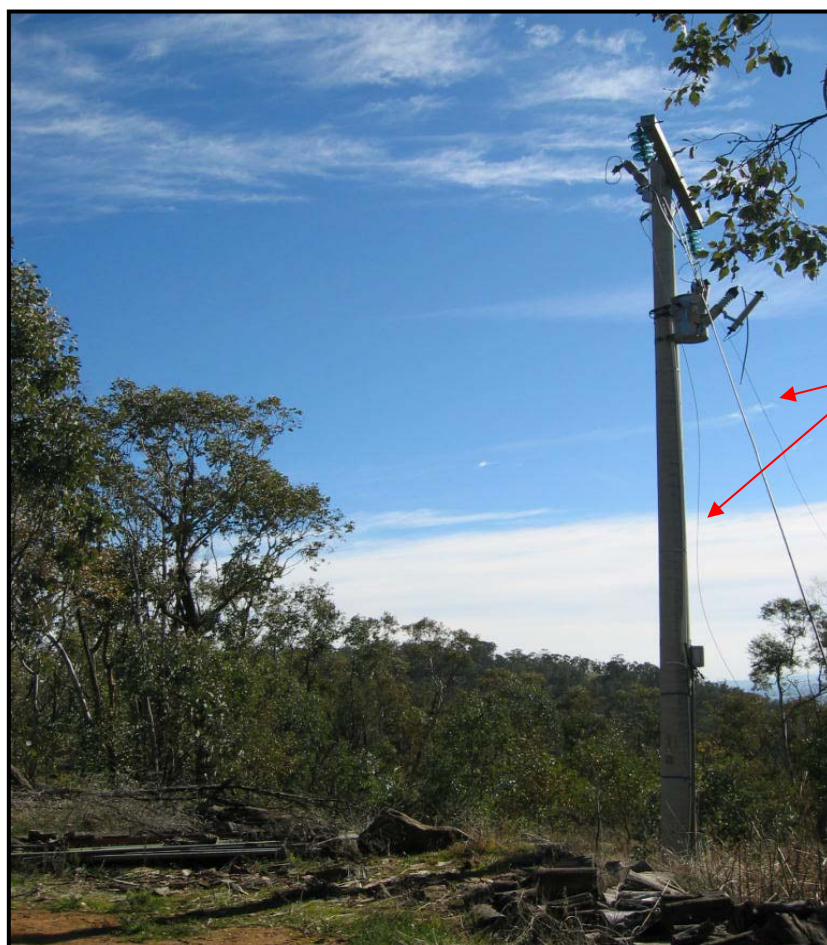
Figure 8: Damaged powerlines after being struck by the Bell 47G-3B-1 Soloy helicopter
