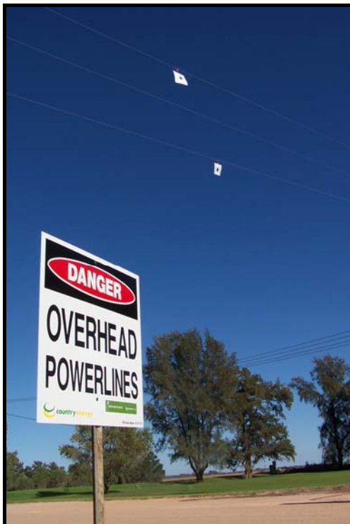
Figure 17: Example of a ‘flag marker’ used on overhead powerlines
