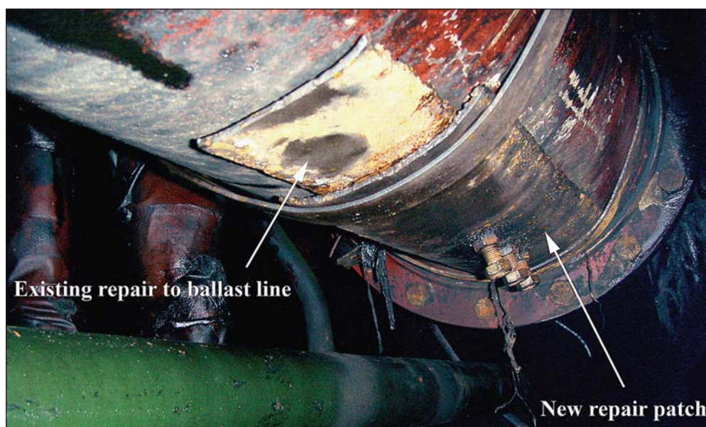
FIGURE 6: Area of leak and patch
