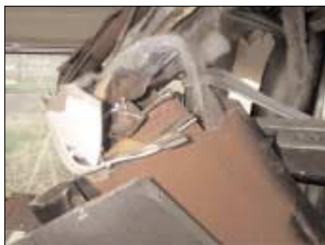
FIGURE 7: Left Hand and right hand collision post failures car 334 M
