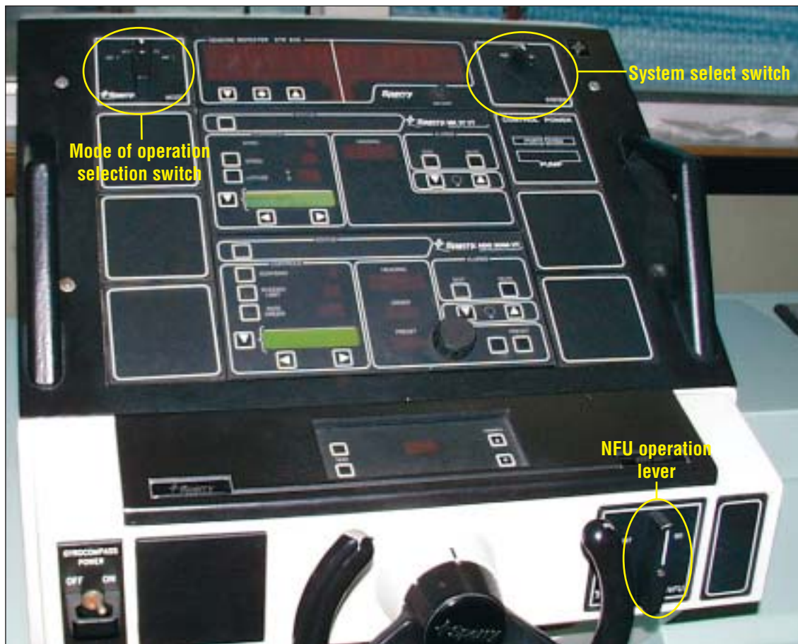
FIGURE 3: Steering motor control panel
