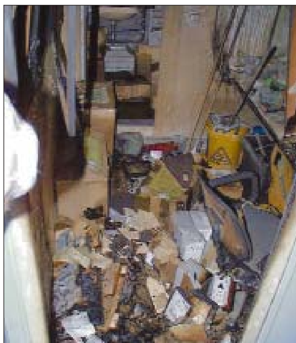
FIGURE 6: Fire debris in the forward section of the store
