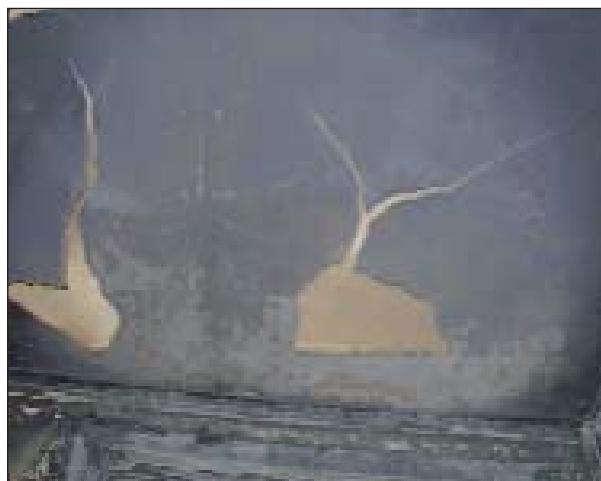
FIGURE 5: Heat damage to deckhead panelling
