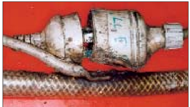
FIGURE 9: The features of the recovered section of the electrical lead and drain hose (two views)
