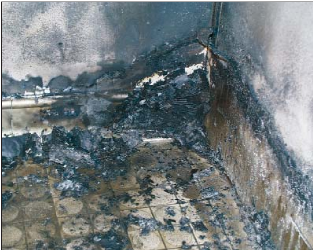
FIGURE 8: Fire damage under computer workstation showing 'V' pattern in corner
