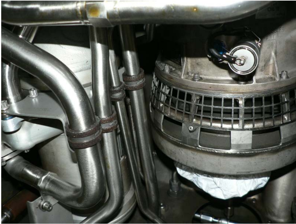
Figure 3: Starter and adjacent oil and fuel lines
