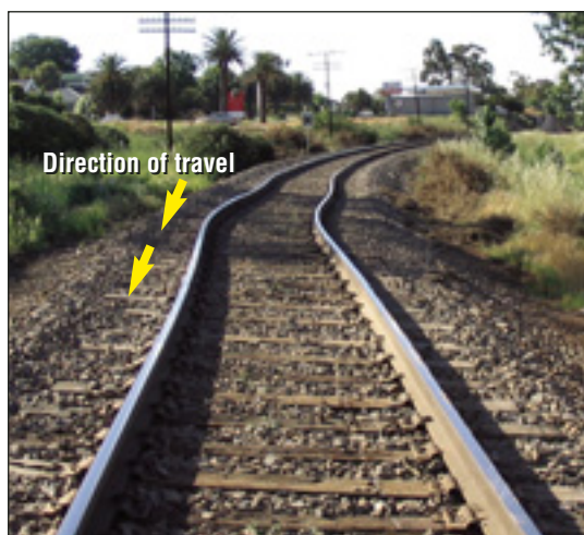
FIGURE 1: The buckled rail at Ararat looking towards Adelaide
